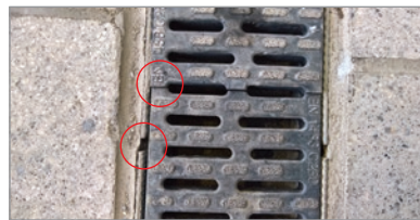
If your inastallation requires the channel to be cut or mitred, ensure the grate still aligns with the anti-shunt. Photo shows a bad installation where the grate overlaps the channel junction
