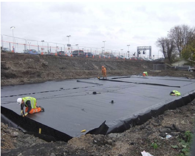
The space-saving benefits of ACO StormBrixx have helped contractors successfully complete the challenging groundworks phase of the Didcot Parkway Station redevelopment.
