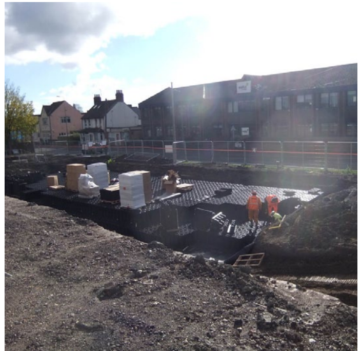
To avoid installation delays, all ACO StormBrixx components were kept on site thanks to its stackable body.
