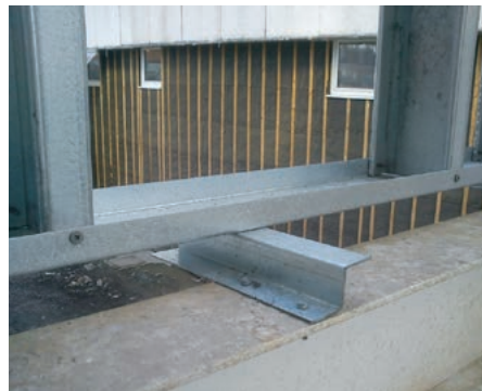
Figure 9.2 Z bar support brackets to infill walls along the line of the edge beam
