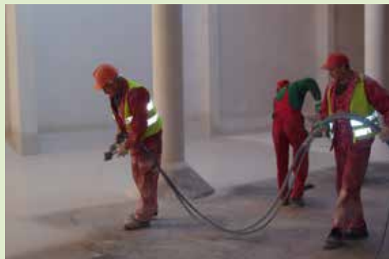
Drinking water tank, Tarnów, Poland
