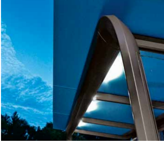
LED lights softly illuminate the inside surface of the roof and provide directional lighting for entrance and egress.
