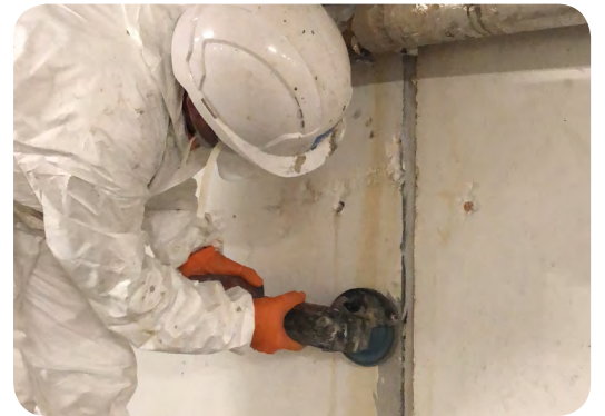
1. Grinding paintwork from concrete to create a good key for the Newton 106 FlexProof
