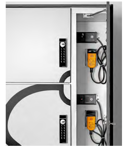
powerBox service compartment for maintenance
