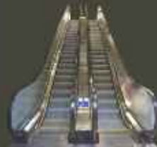
Escalators and Moving Walkways
