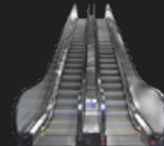
Escalators and moving walkways
