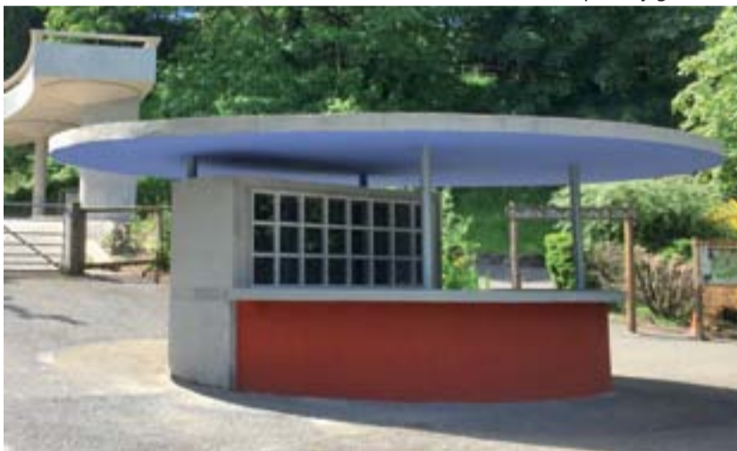
The ticket kiosk was originally constructed without any waterproofing protection at all.
