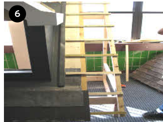
6 Gauge the rest of the tiling battens between critical top tile and eaves tile as appropriate for roof pitch and tile
