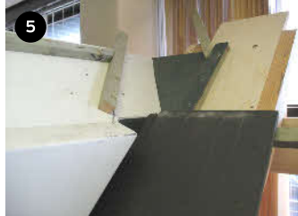
5 Top tile will now be in a position at the base of valley making the lead saddle run straight (without any kinks) onto the tiles
