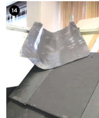
14 Cut valley tiles according. Bed as necessary onto GRP valley tray or on to cloaking piece placed onto lead. Ensure a drainage channel is kept behind mortar bed.
