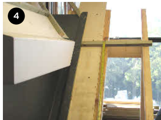
4 As with a traditional chimney, set out critical batten at top of dormer. Set batten level with bottom of valley
