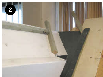
2 Set counter laths 150mm each side of centre of valley. Abut tiling battens into counter lath with nominal gap. A 6mm lay board should be fitted to support lead or proprietary valley gutter as per traditional detail. (Lay board not shown)
