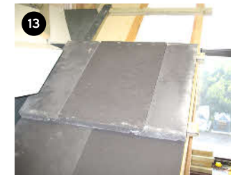
13 The tiles should now course evenly with the top tile almost level with the valley
