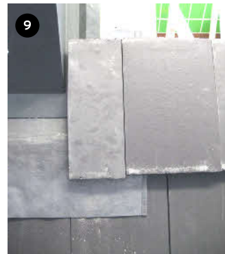
9 Using full and half tiles (tile and half preferred) set tiles within a maximum of 15mm from side of dormer. This inside tile now covers foam
