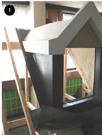
1 Position dormer on roof according to window head and cill levels required. Fix as per standard details.
