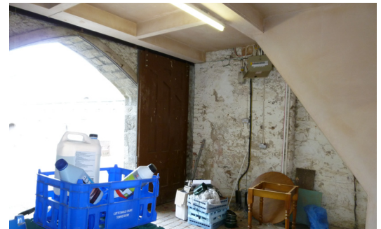
The walls in this outbuilding were affected by penetrating damp and had structurally degraded
