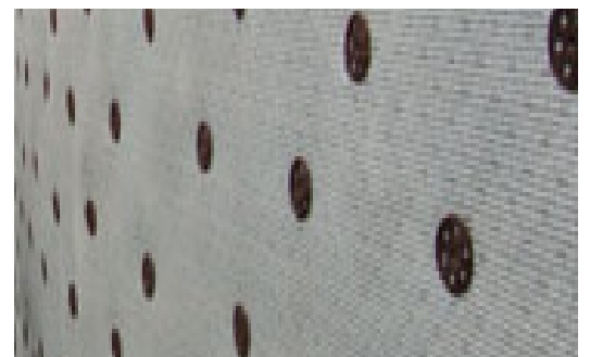
Newton 805 Newlath was ideal for treating the damp walls as it conformed with Listed Building requirements
